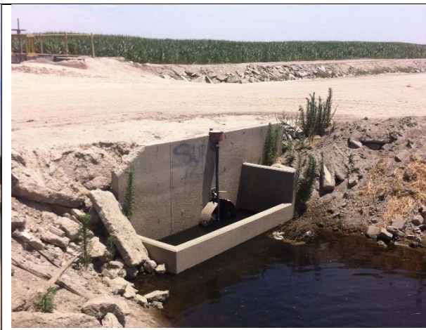
Typical open-flow meter installation. Note the weir wall placed to keep the pipe full.
