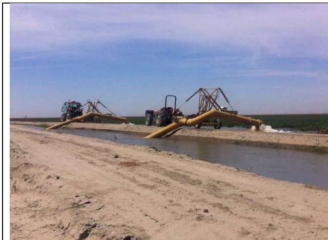
Typical mobile pumping system.
